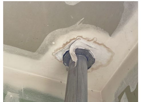
Water heater closet
